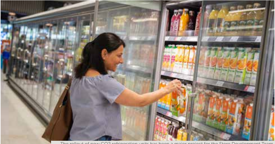
The rollout of new CO2 refrigeration units has been a major project for the Store Development Team.
